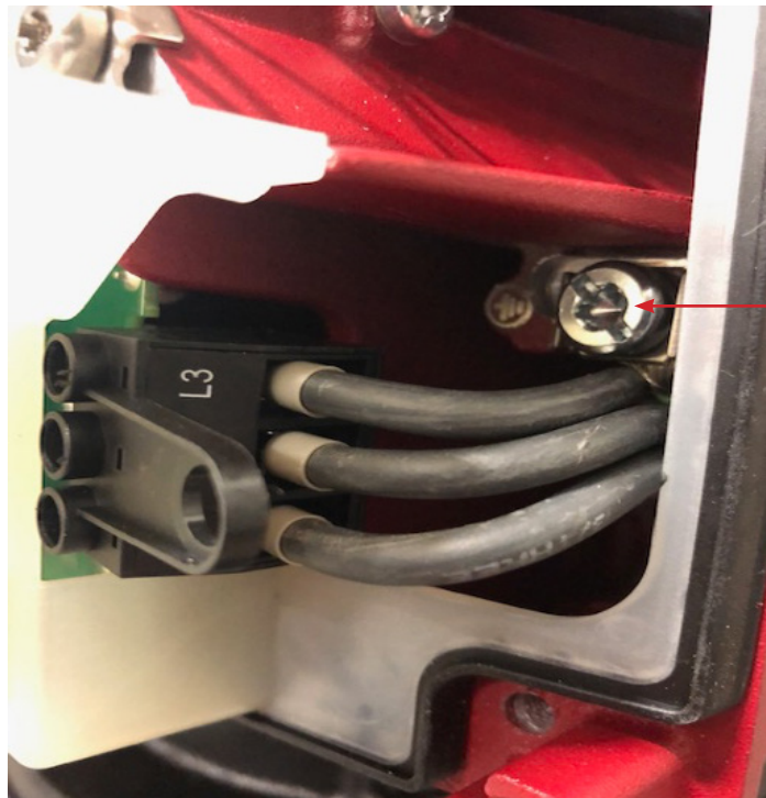
Fig. 3.3 - 2 - Pump grounding conductor and ground lug
