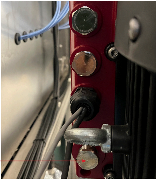
Fig. 3.3 - 1 - Pump 3 PH incoming power connection
